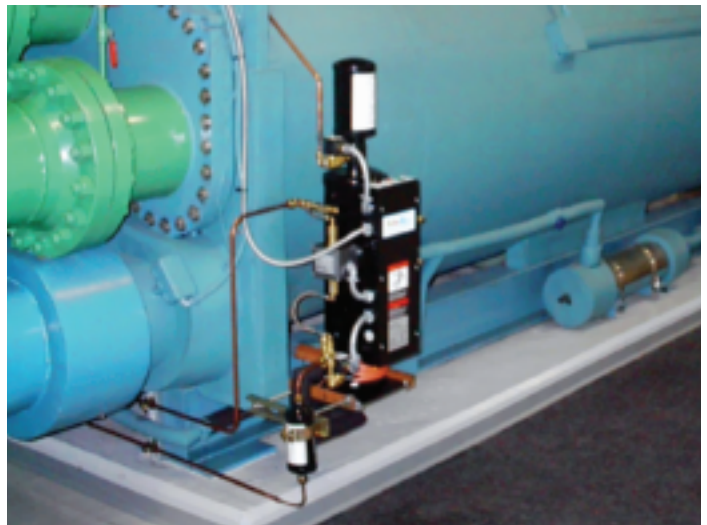
The chiller's performance degraded from 0.89 kW/ton to between 1.1 and 1.5 kW/ton.
