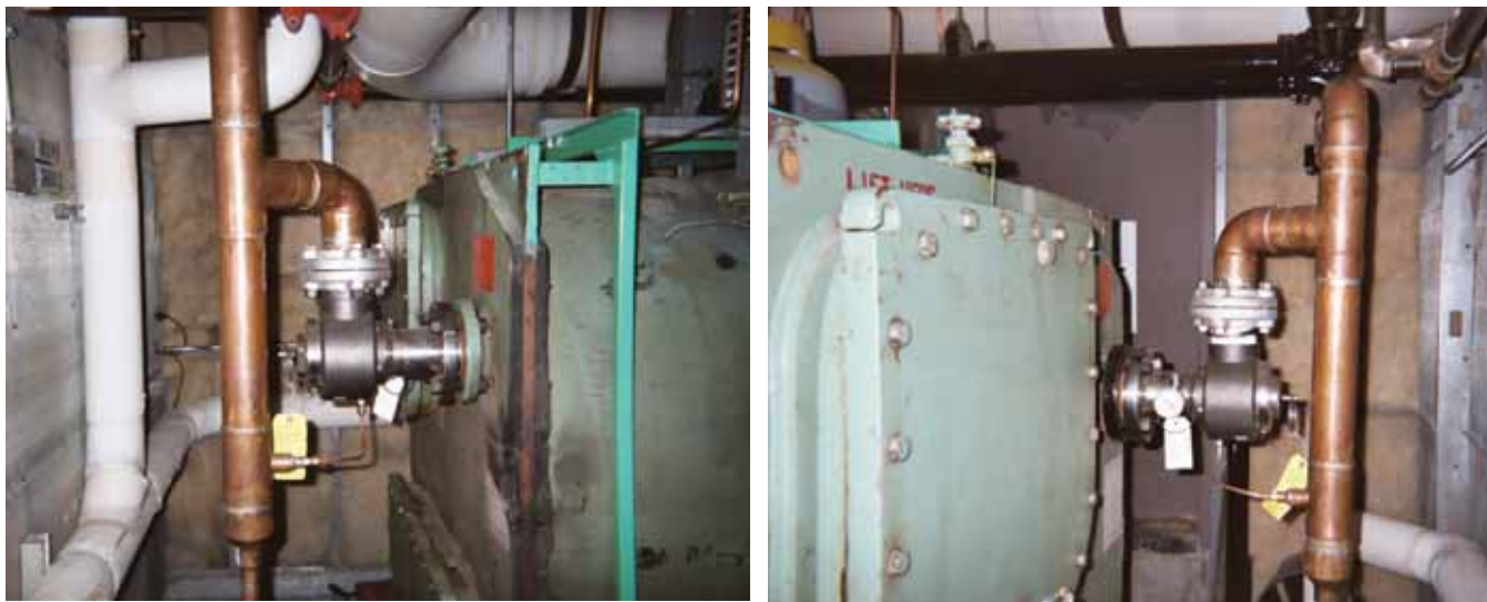
Photos are of the RuptureSeal Model NRS-2 backup safety relief valves for low pressure centrifugal chillers installed by Johnson Controls Alaska at the BP and Frontier Group facilities.
