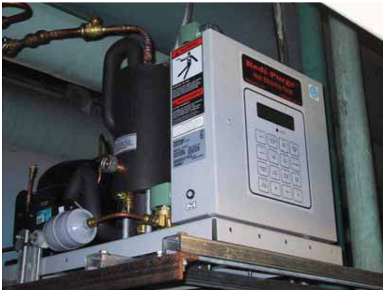
Photo of a Redi-Purge Model PRG-11/123-C2 ARI Certified UL Listed High Efficiency Non-Condensable Purge installed at Complex LaLaurentienne Canada.
