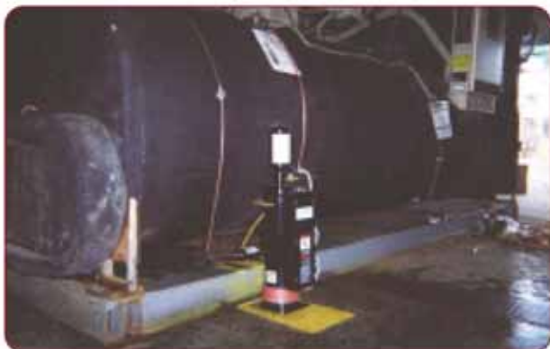
OAM Purger installed at the 3M facility, Buffalo, NY
